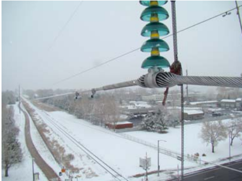
Platte River Power installation with 3M ACCR suspension assembly, bike path on left and railroad track on right.
